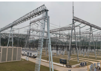
Electricity power inspection
