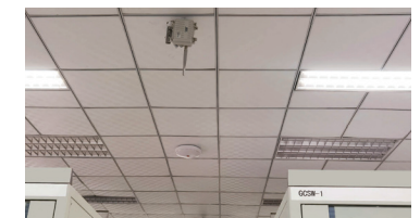
UWB base station installation
