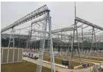
Electricity power inspection
